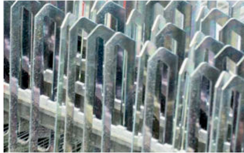
Prior to cleaning
